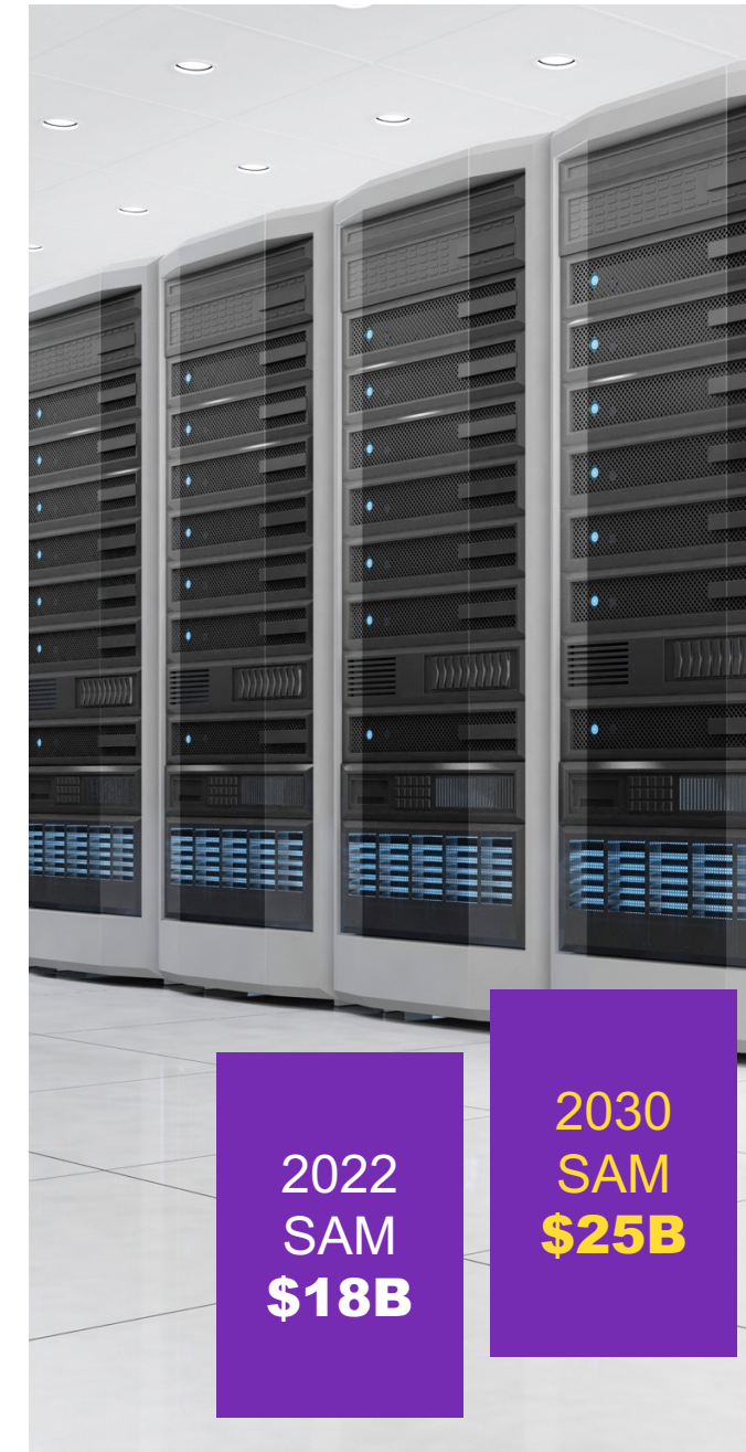
Communications Infrastructure & Datacenter
